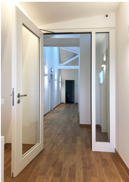
▲ POLFLAM ® fire-resistant glass was installed in woodwork at a Luxembourg minister's office
